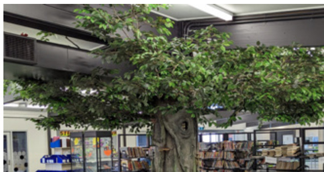
After installation, the tree's foliage helps to conceal the ducting
